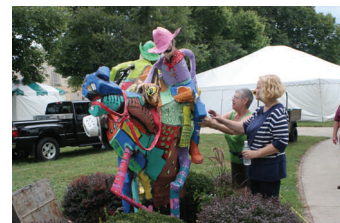
Volunteers Barb Crumley and Vicki Christgen make repairs to the Trails West!® statue.
